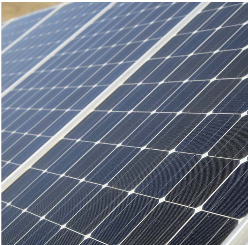
Image of a solar photovoltaic (PV) installation
