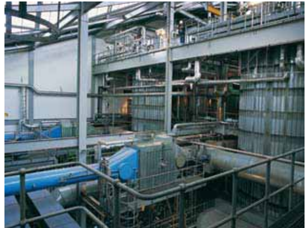
Thames Water sewage treatment works, sewage incinerator
