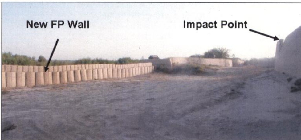
Fig 1-11 The construction of a new FP wall and the impact point of the CH47 on the pre-existing wall
