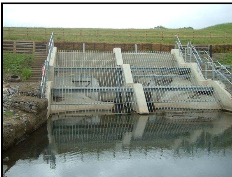
FSA outlet with flow control device and screen
