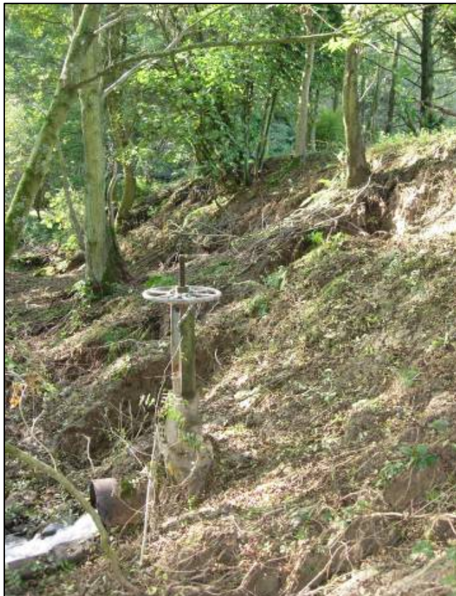
Figure 5.1 This dam was nearly washed away when it was overtopped in 2008.
