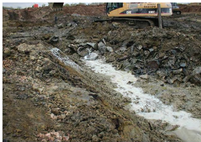
Photograph 2: Recovered damaged drums (©Celtic Walters Land Ltd., 2005).
