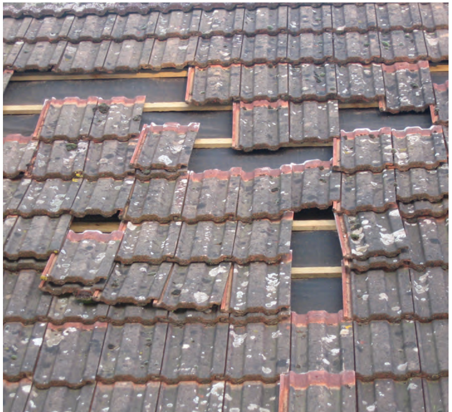
Photograph 1: Photographs of damaged buildings in the vicinity of the fireworks fire and explosion near Lewes (© Health Protection Agency, 2006).
