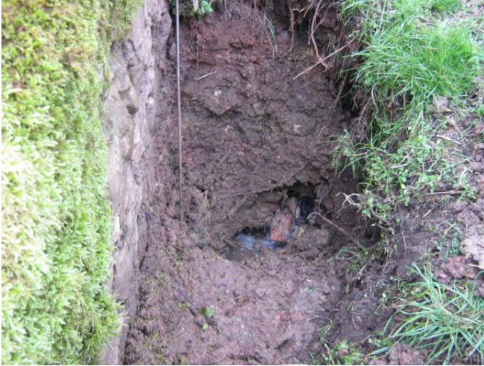
Figure 3.2 Trial hole to investigate the source of the leak (Photo courtesy of Wessex Water)
