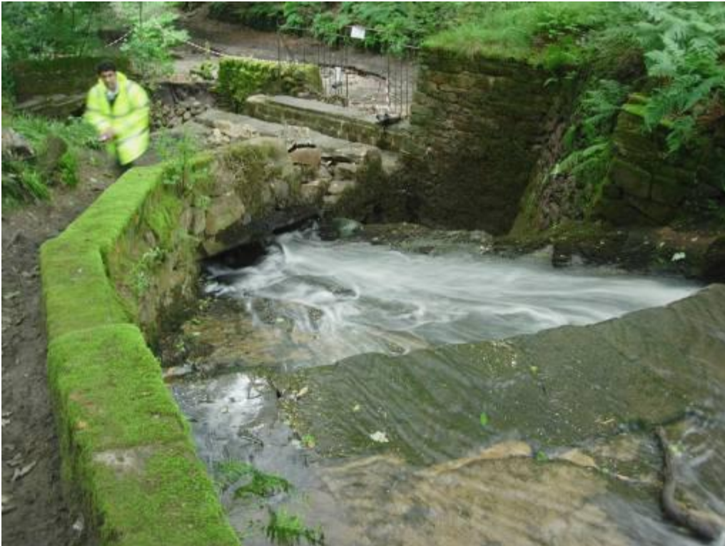
Figure 3.7 Upper reservoir spillway showing damage to the wall (Photo courtesy of Alan Warren)
