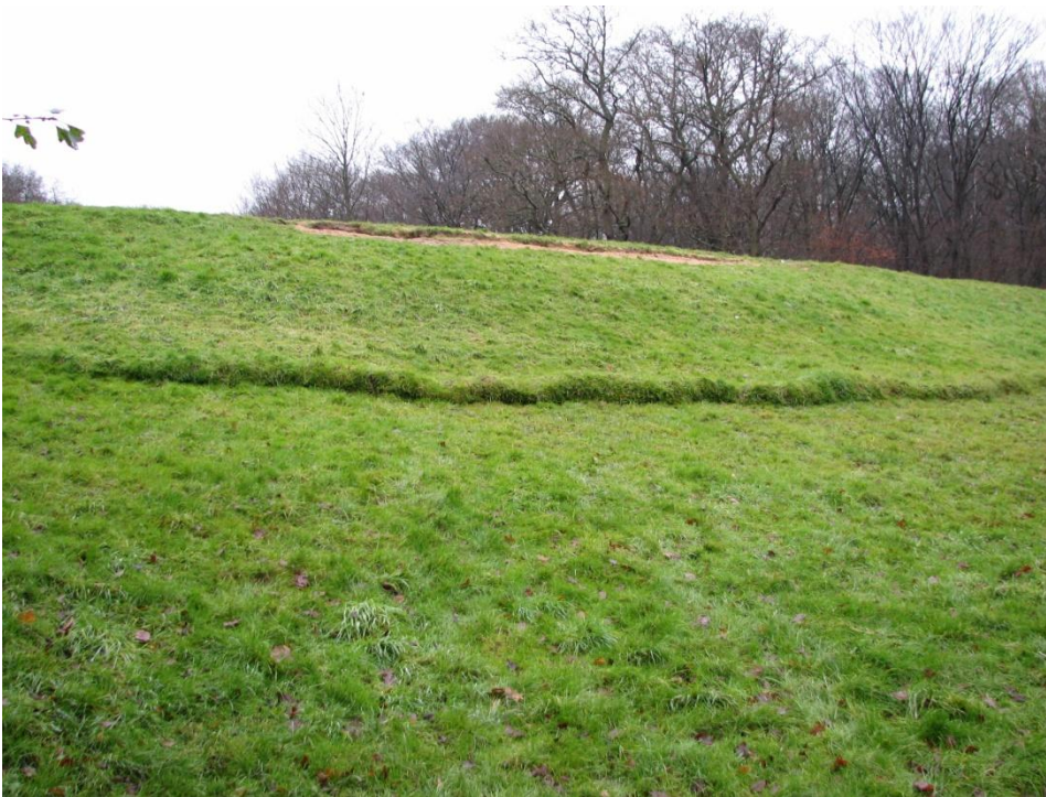
Figure 3.14 Instability of reinforced topsoil layer on the embankment downstream face (Photo courtesy of Andrew Pepper)
