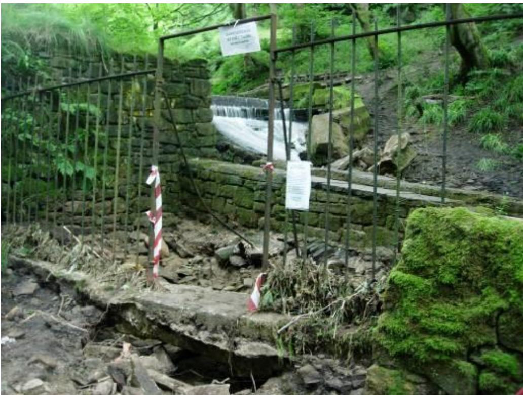
Figure 3.8 Damage to the overshoot channel of the upper reservoir (Photo courtesy of Alan Warren)
