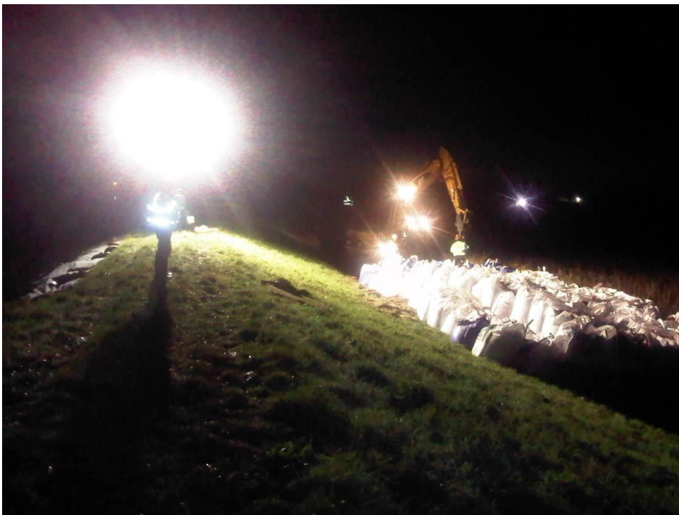
Figure 3.12 Emergency works to stabilise the slope (Photo courtesy of John Falkingham Associates)
