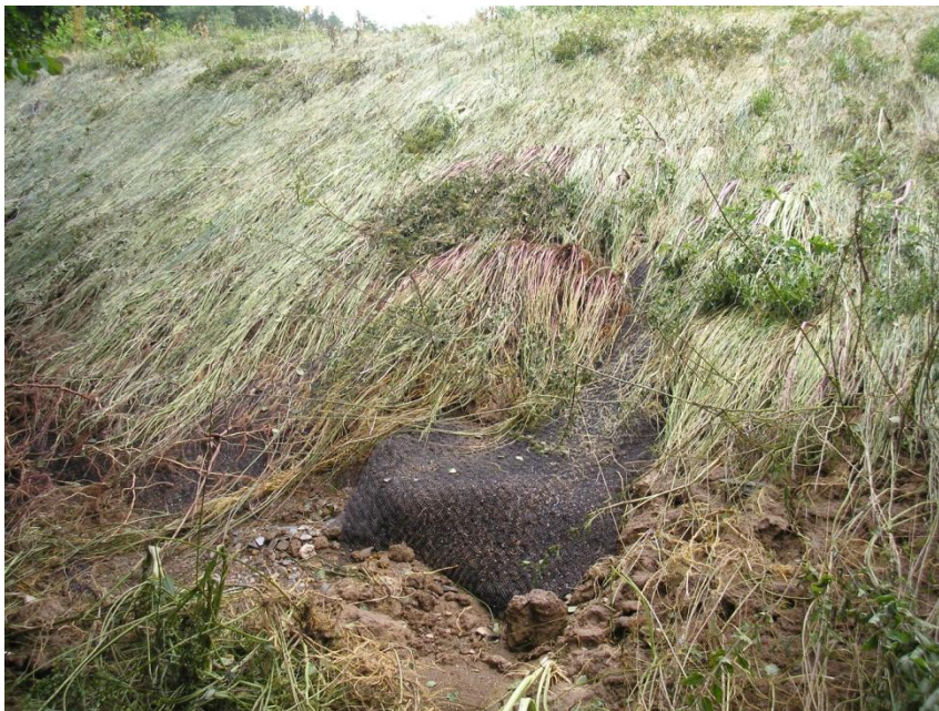
Figure 3.10 Scour damage at the downstream toe (Photo courtesy of Richard Cox)
