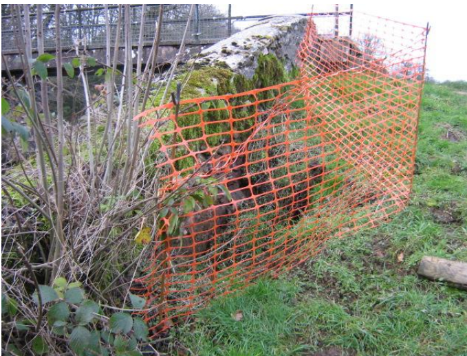
Figure 3.1 Sink hole beside the spillway wall (Photo courtesy of Wessex Water)
