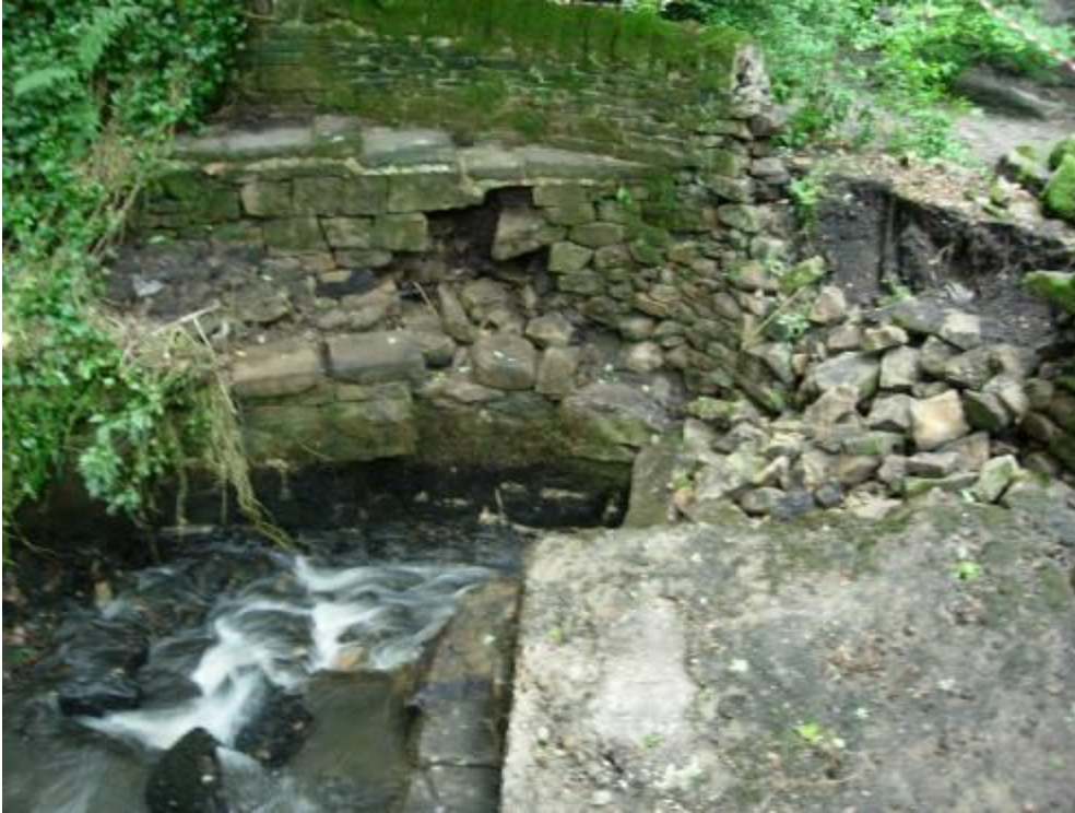
Figure 3.9 Damage to the upper reservoir stilling basin (Photo courtesy of Alan Warren)
