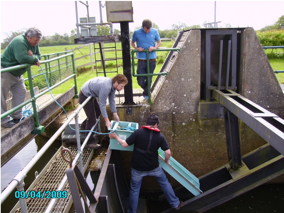
Figure 2.4 Siphon-fed trap being fitted on anchor-tilting weirs, Sussex Ouse Picture: Sally Chadwick
