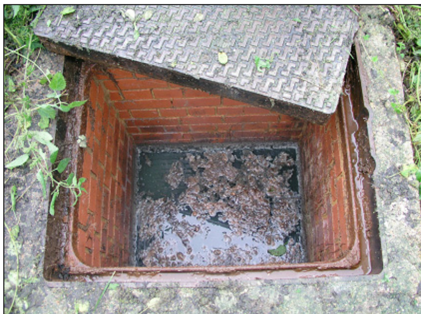
Figure 7.4 Holding tank C3.
