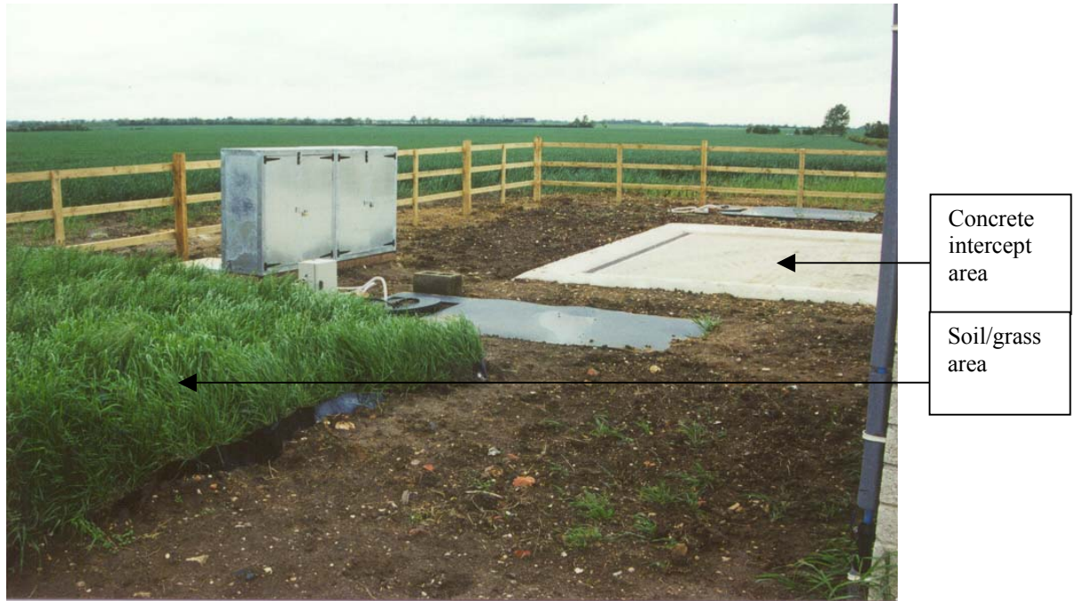
Figure 4.6: Concrete intercept to soil/grass area
