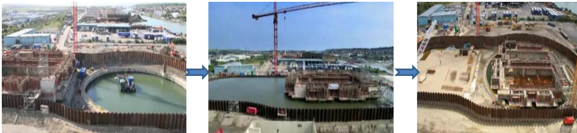
These photographs show the phased construction of the ERF plant on a raised platform, which was then floated into position and 'sunk' into its foundations 68
