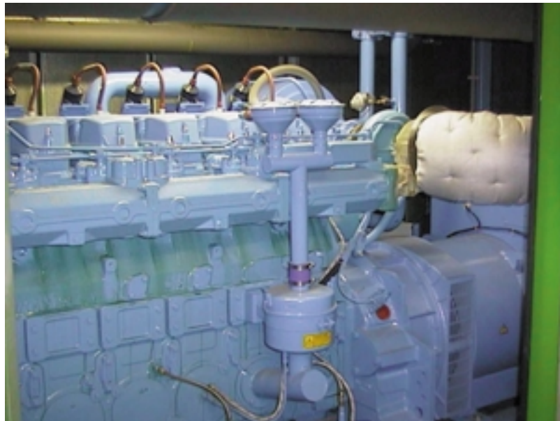
NEDALO CHP PLANT AT LAGAN VALLEY HOSPITAL SHOWING GENERATOR INSIDE ACOUSTIC HOUSING: PHOTOGRAPH COURTESY DOWN LISBURN TRUST
