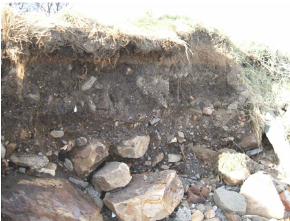
Plate 3: Damage and Erosion to Area Formerly Protected by Rock Armour
