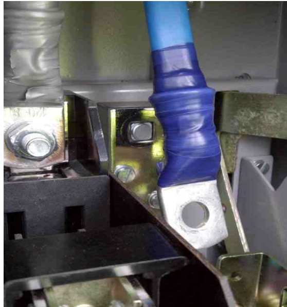
Fractured Terminal Bolt
