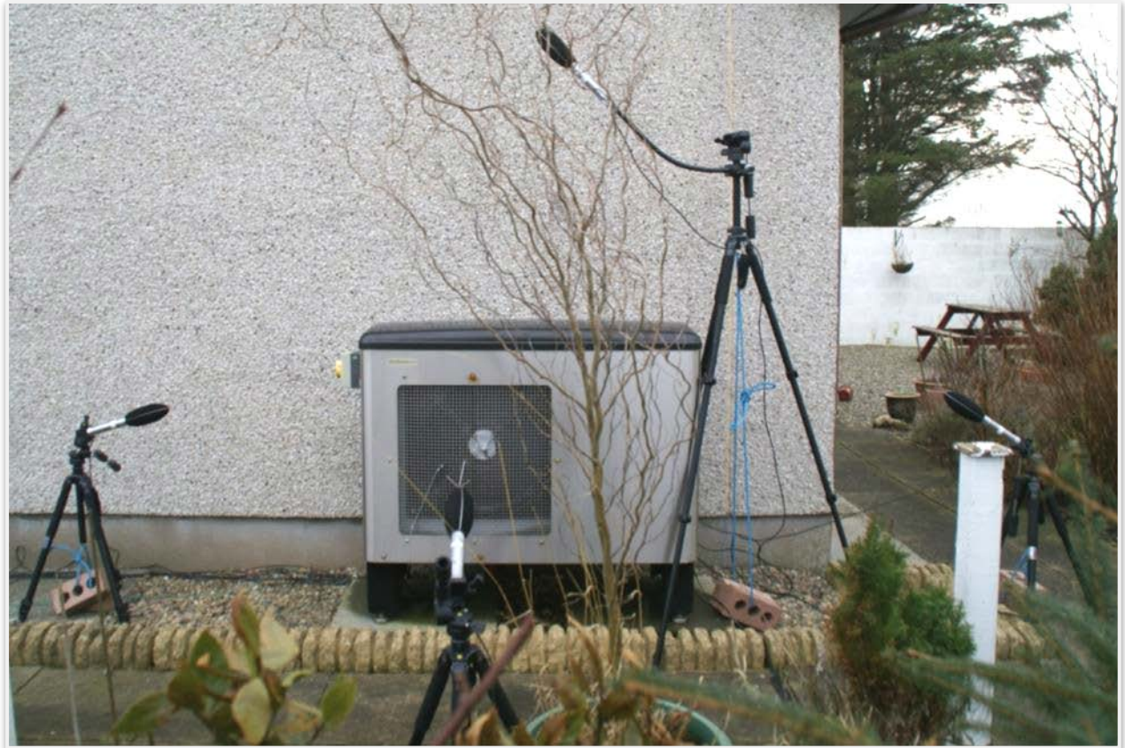
Picture 5-12. 422 Fraserburgh, Original ASHP and Microphone Arrangement
