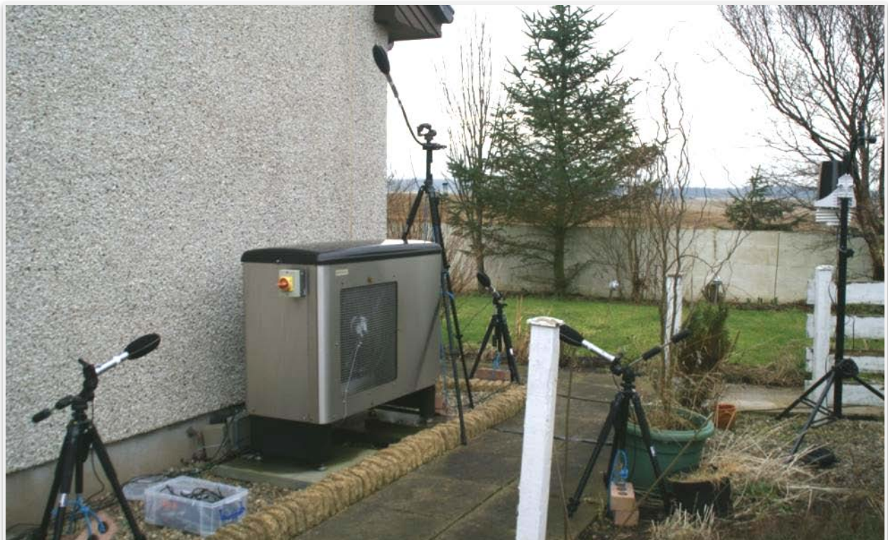
Picture 5-11. 422 Fraserburgh, Original ASHP and Microphone Arrangement
