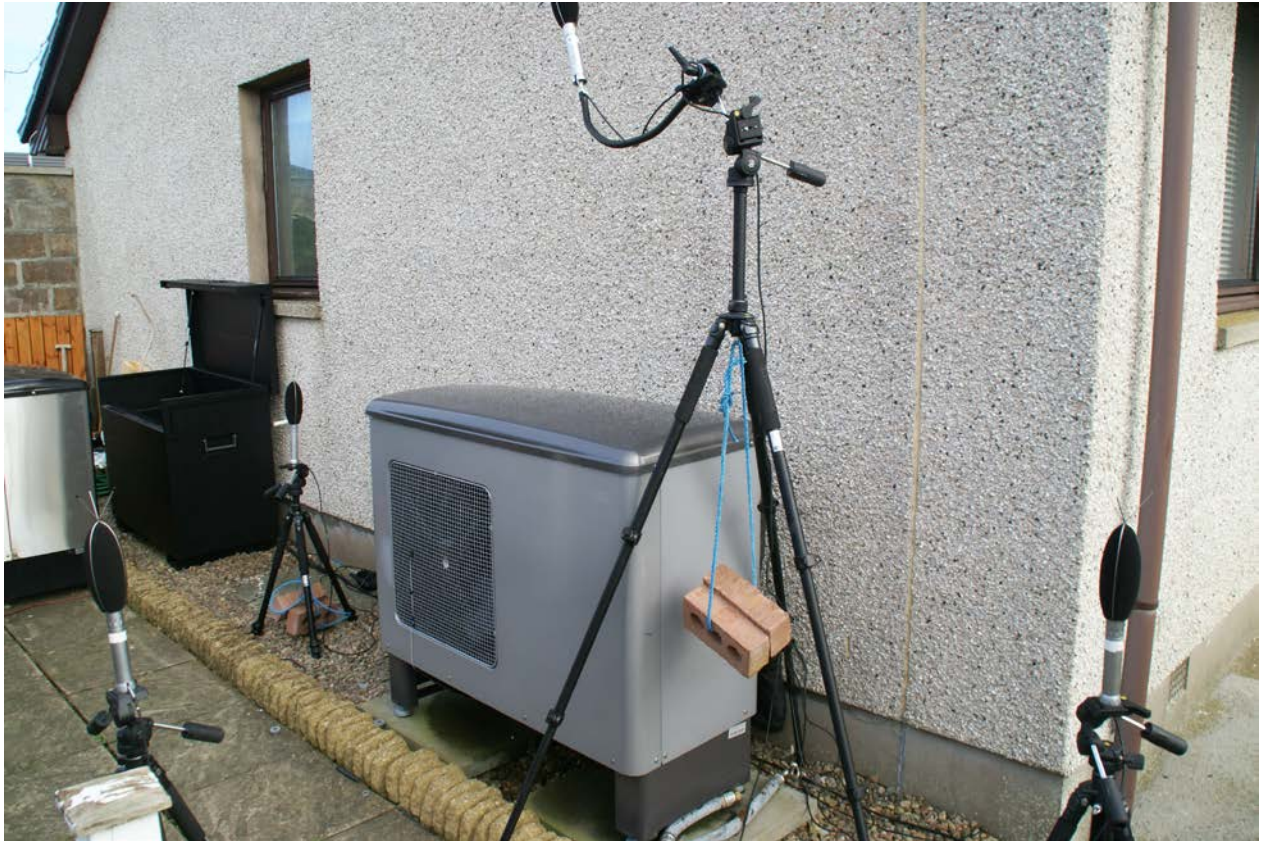
Picture 5-14. 422 Fraserburgh, Replacement ASHP and Microphone Arrangement
