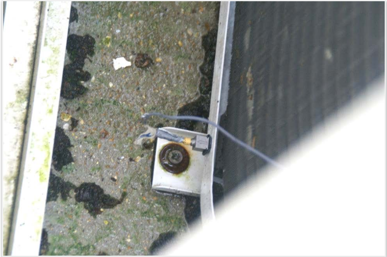
Picture 5-17. 474 West Berkshire (Site 1), Casing-mounted Accelerometer
