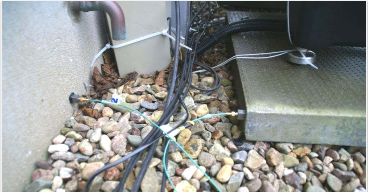
Picture 5-10. 422 Fraserburgh (Original), Footing and Wall-mounted Accelerometers
