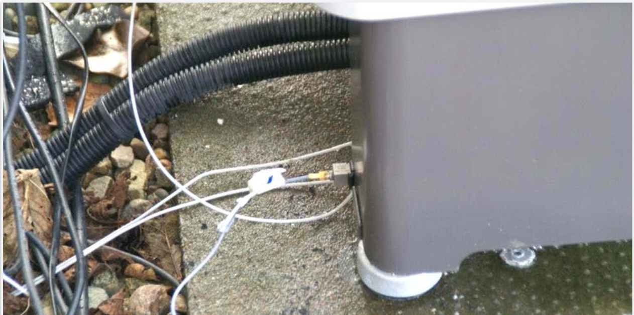
Picture 5-13. 422 Fraserburgh (Replacement), Casing-mounted Accelerometer
