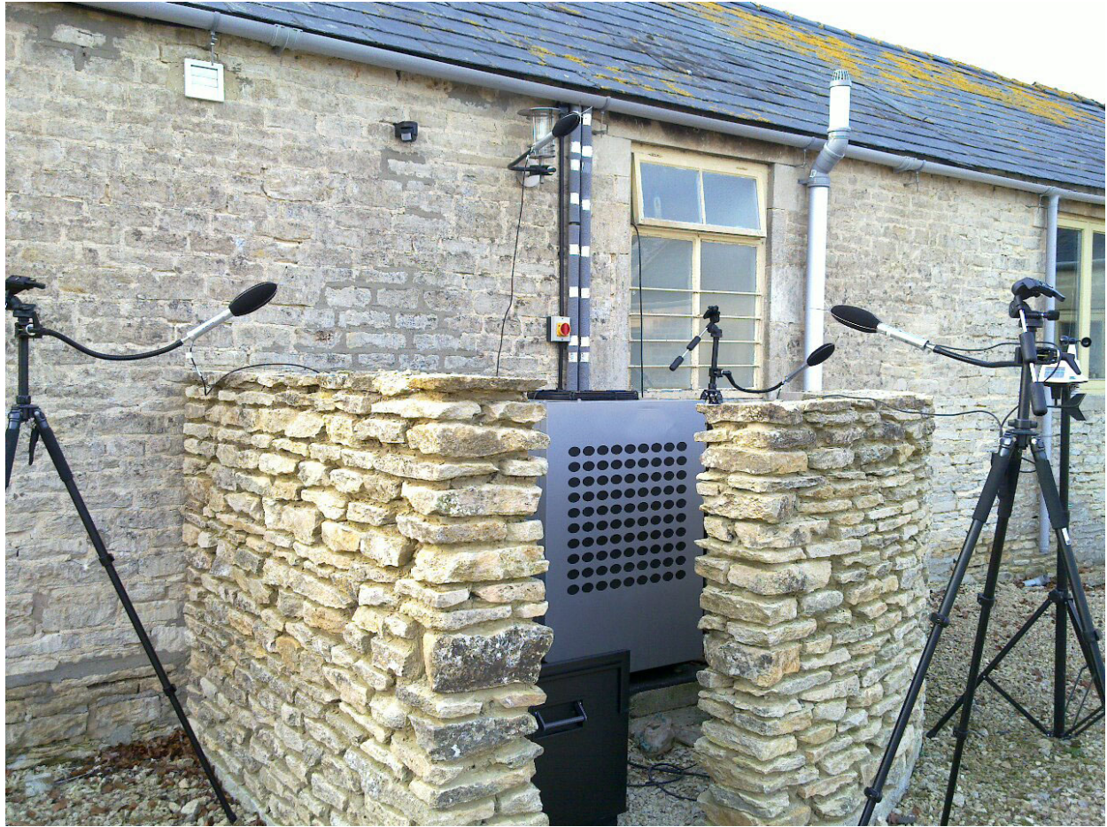
Picture 5-23. 478 Cotswold (Courtyard), ASHP and Microphone Arrangement
