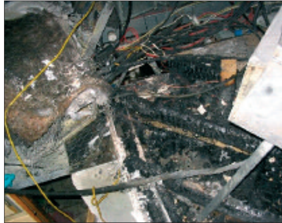
Figure 18: Station fire (courtesy of Network Rail)
