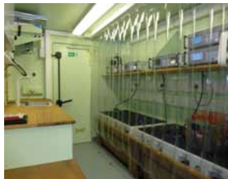
In charge: battery charging facilities for the RAF supplied by Marshall
