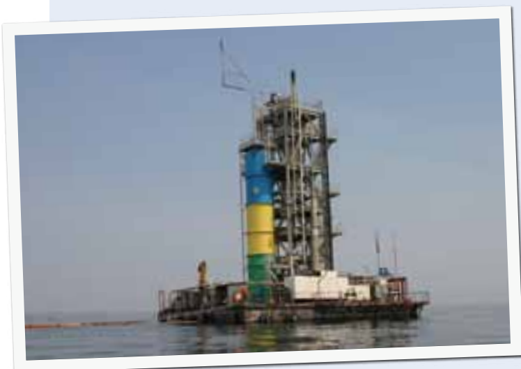
Methane Plant at Lake Kivu
