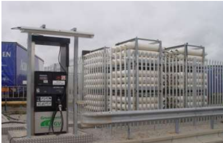
■ Figure 18 Gas storage and CBM Dispenser
