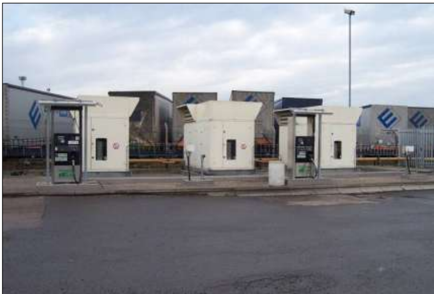
■ Figure 16 CNG-CBM Compressors
