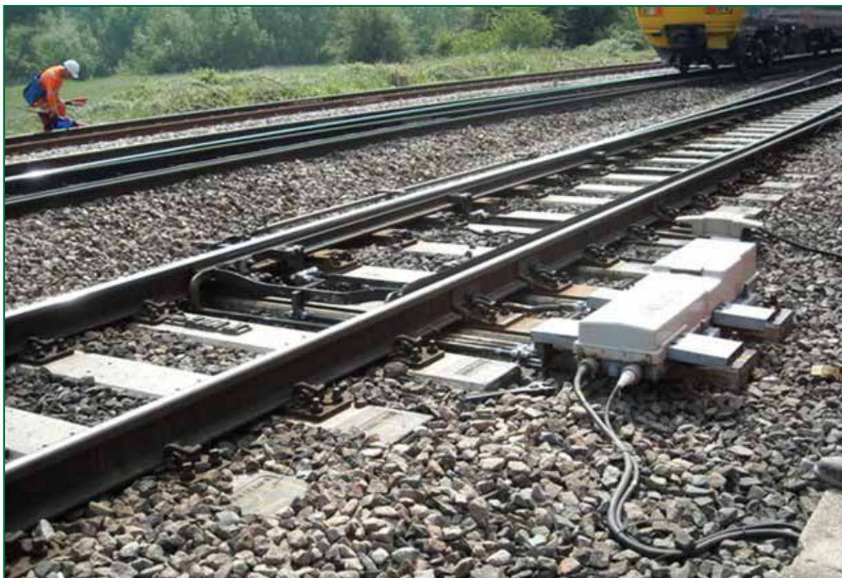
Figure 6:207A point machine. The down line is closest to the camera (Photo courtesy of Network Rail)
