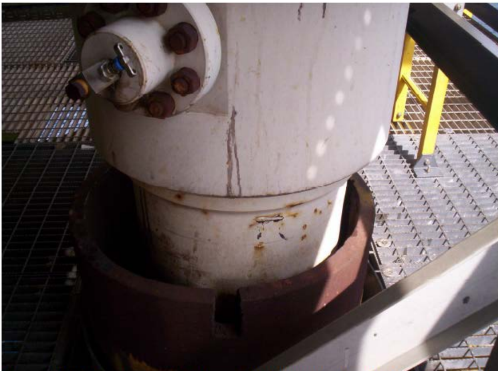
Figure 3-1: Top of Conductor GYA-02 at the South side of the well, showing the 20" Casing leaning towards the South-East
