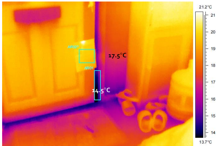
Figure 45: Thermal image of the front door and hallway in D10
