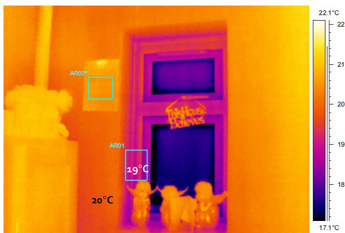
Figure 47: Thermal image of the hallway of property D10
