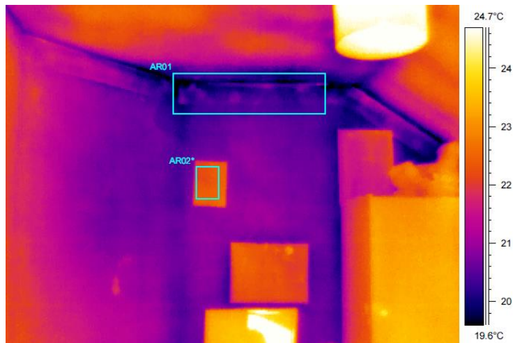
Figure 14: Thermal image of the back bedroom of D3
