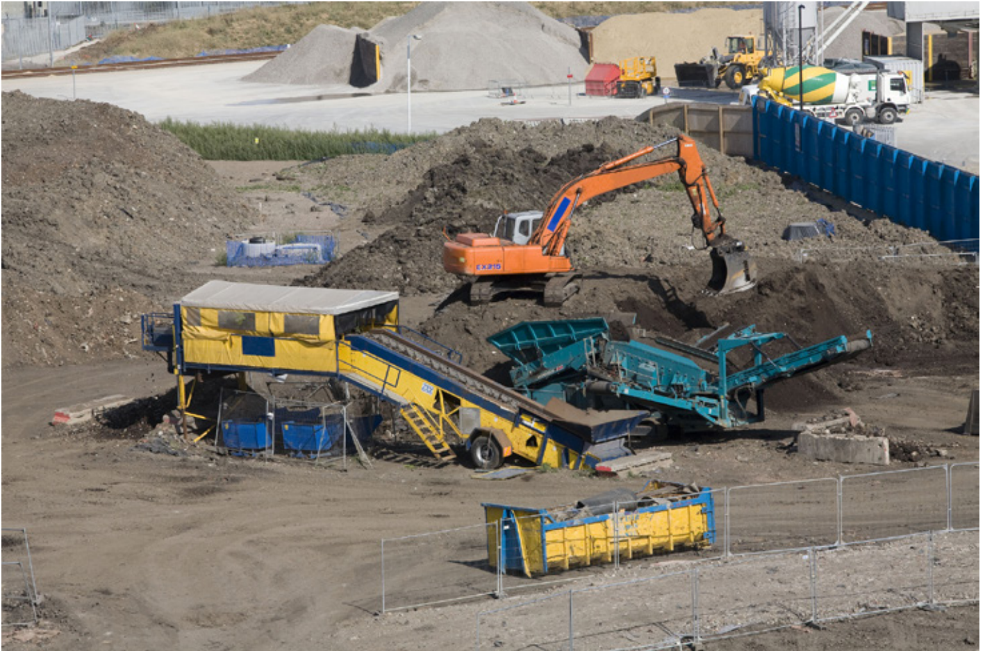
Soil washing with the wider aim of bioremediation at the Olympic Park.
