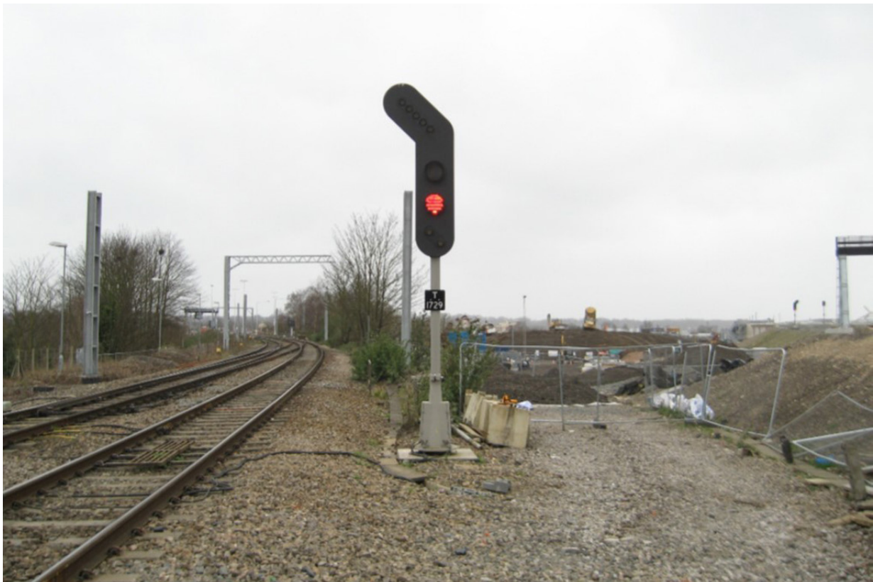
Figure 2: Signal T1729 at Reading Westbury Line Junction (image courtesy of DB Cargo (UK) Ltd)
