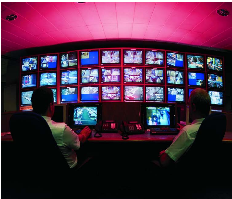
Image: CCTV Control Room Copyright © Centro
