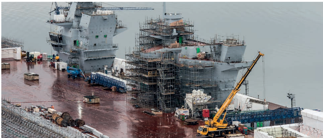
The aircraft carrier HMS Queen Elizabeth under construction at Rosyth Dockyard, Scotland. Whilst the MOD travel policy discourages avoidable business travel, sometimes our people need to be onsite, wherever that may be
