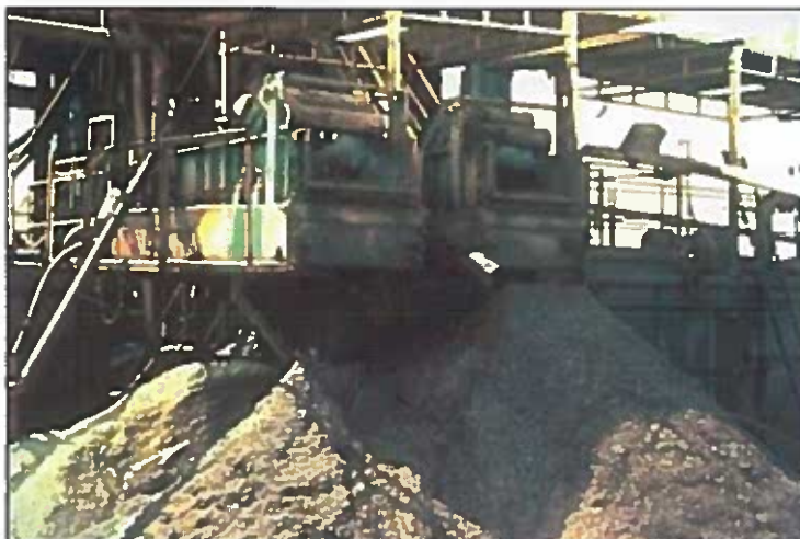
Figure 3-5: Example of an operating shale shaker, with cuttings pile in the foreground.
