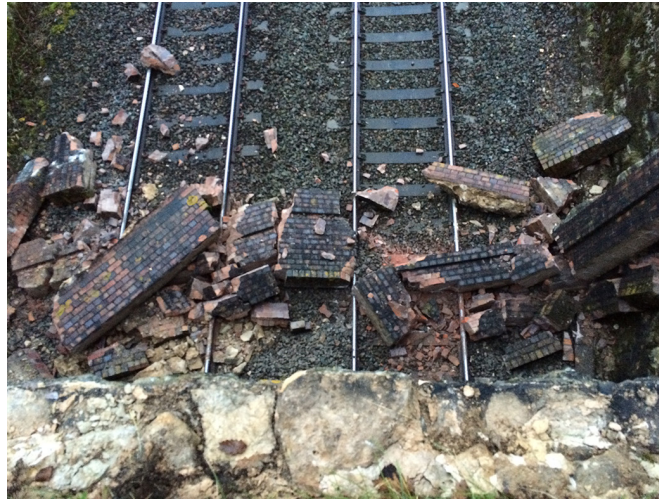
Collision between a train and a fallen bridge parapet near Froxfield (02/2016) (image courtesy of Mr John Brown)
