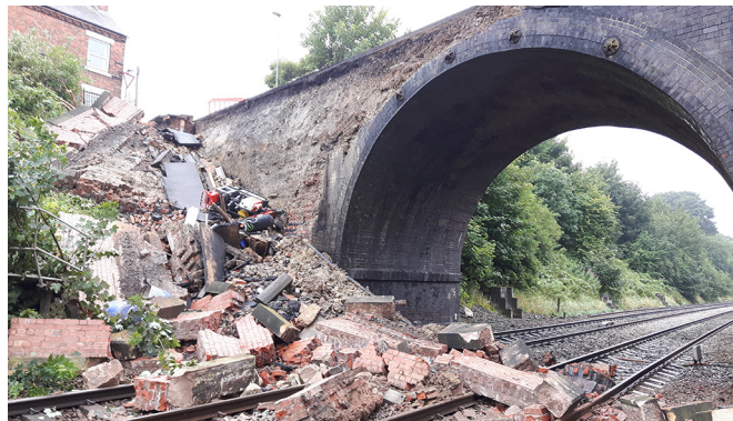
Partial bridge collapse at Barrow-upon-Soar
