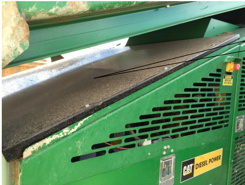
Enclosure over engine compartment
