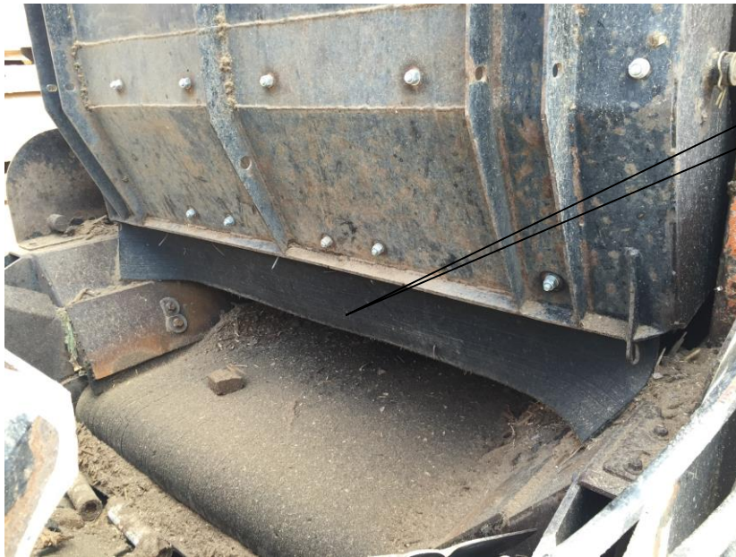
Rubber damping to hammer mill
