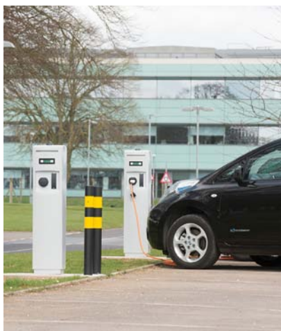
Electric vehicle charging pillars at Dstl Porton Down.
