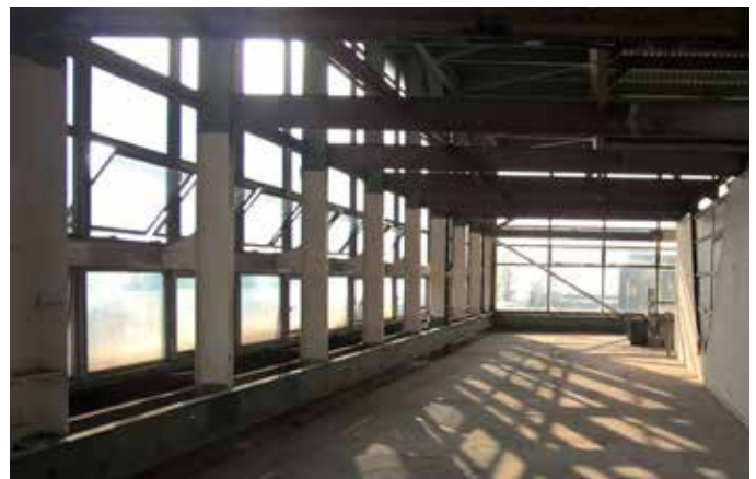
Existing facilities at the Gloucestershire science park are being refurbished and upgraded.
