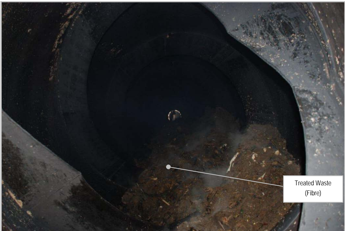
Fig 3.5 & 3.6 . – Waste Recovery Facility – Autoclave Internals pre and post steam sterilisation
