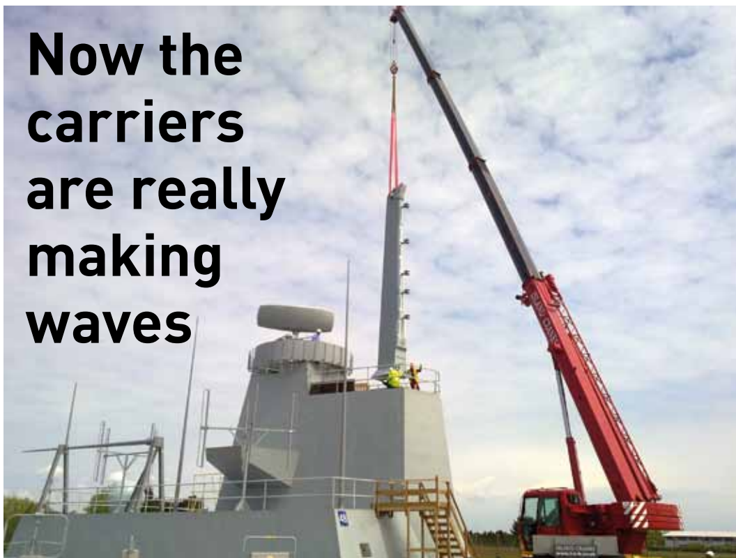
Coronet Building at Cowes is pictured with Artisan 3D as the pole mast is fitted
