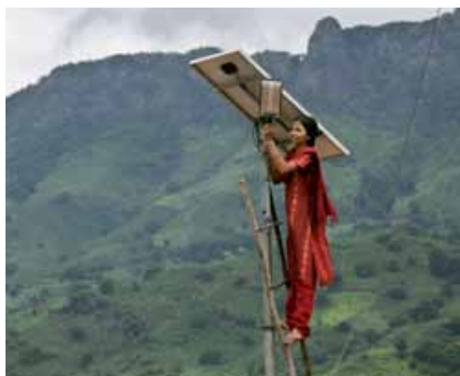
A woman tends to maintenance of solar street lighting in her village in India (Abbie Trayler-Smith/Panos Pictures/DFID)
