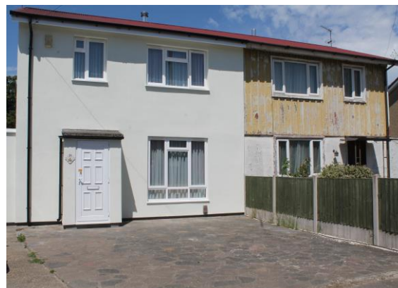
A BISF type system-built home from the 40s externally insulated alongside its neighbour
