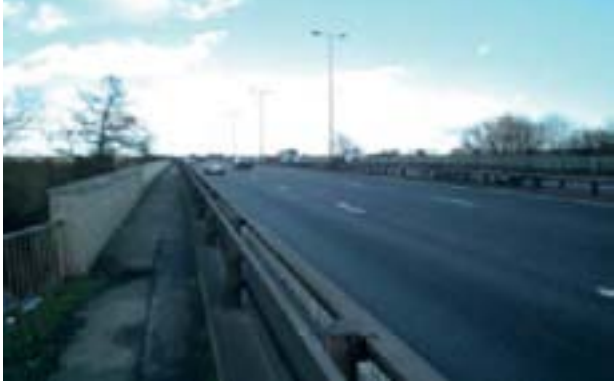
Figure 6: Discontinuous hard shoulder at underbridge
