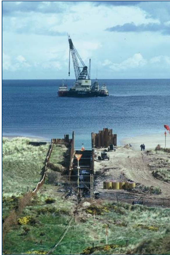
Figure 3.3 - Pulling the first North Sea pipeline ashore at Cruden Bay from the Forties Field in 1973
