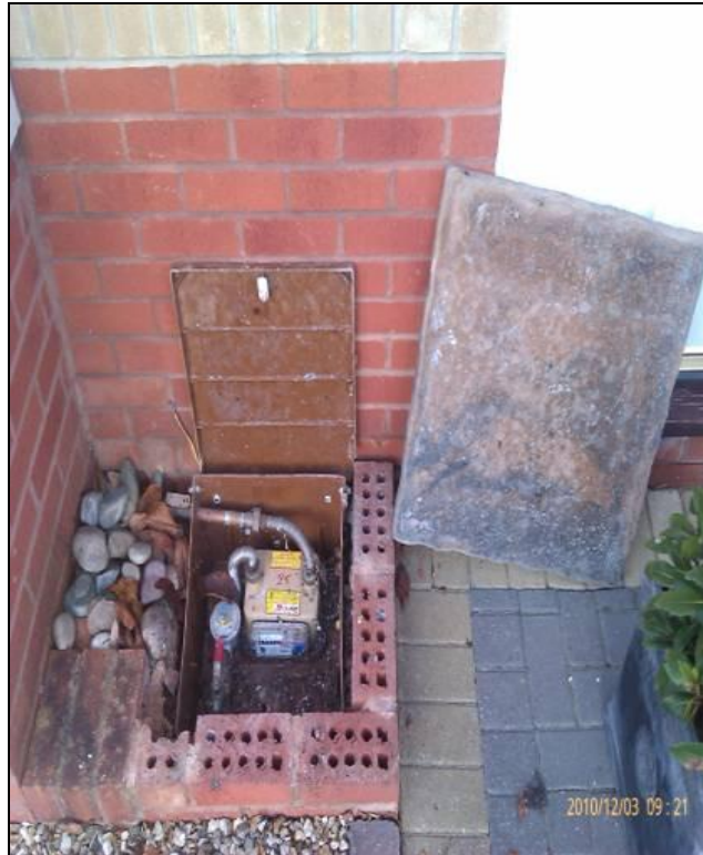
Figure 16: Example of a semi-concealed gas meter
