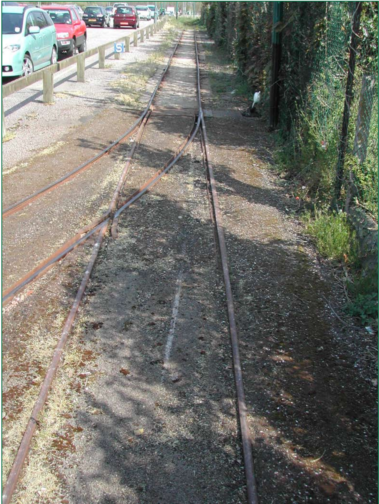
Figure 6: Marks from derailment
