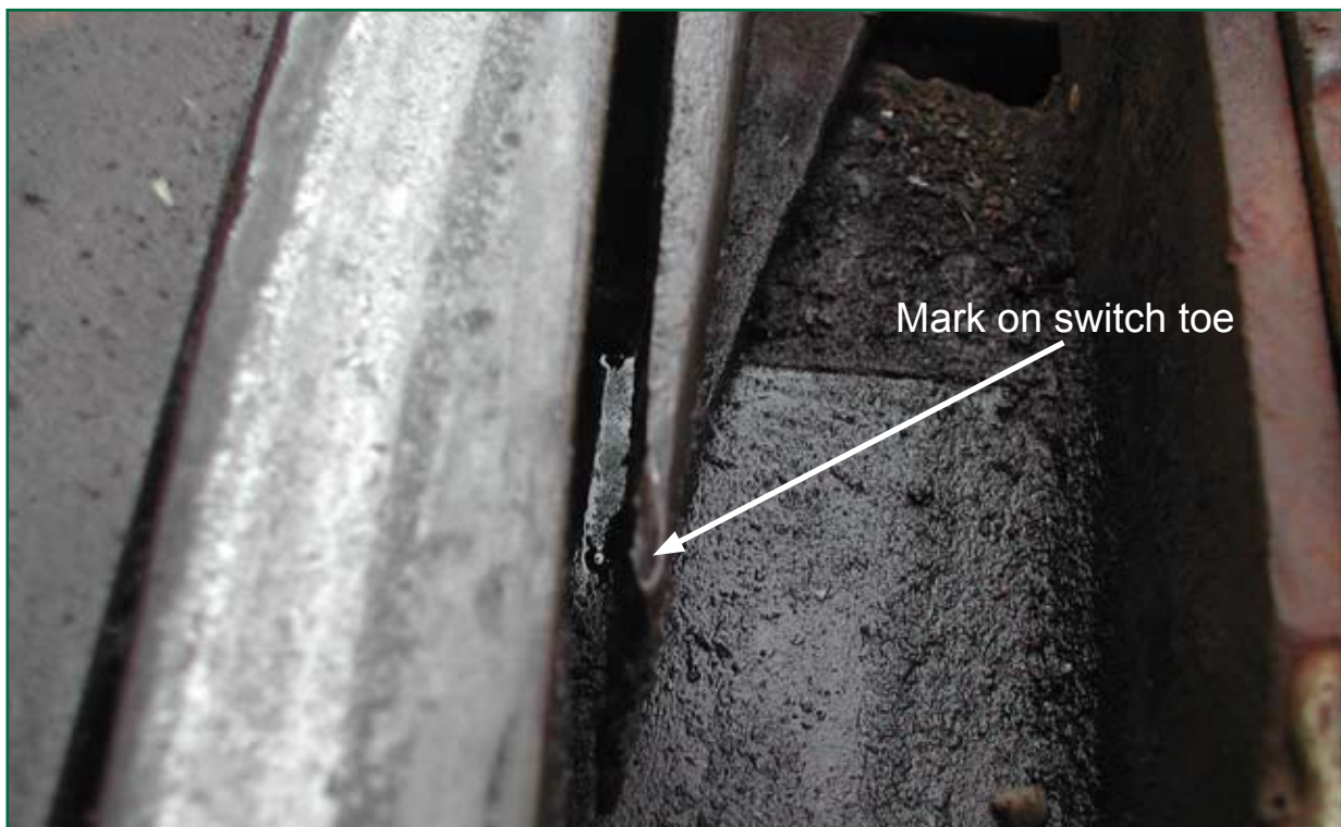
Figure 7: Mark on switch toe
