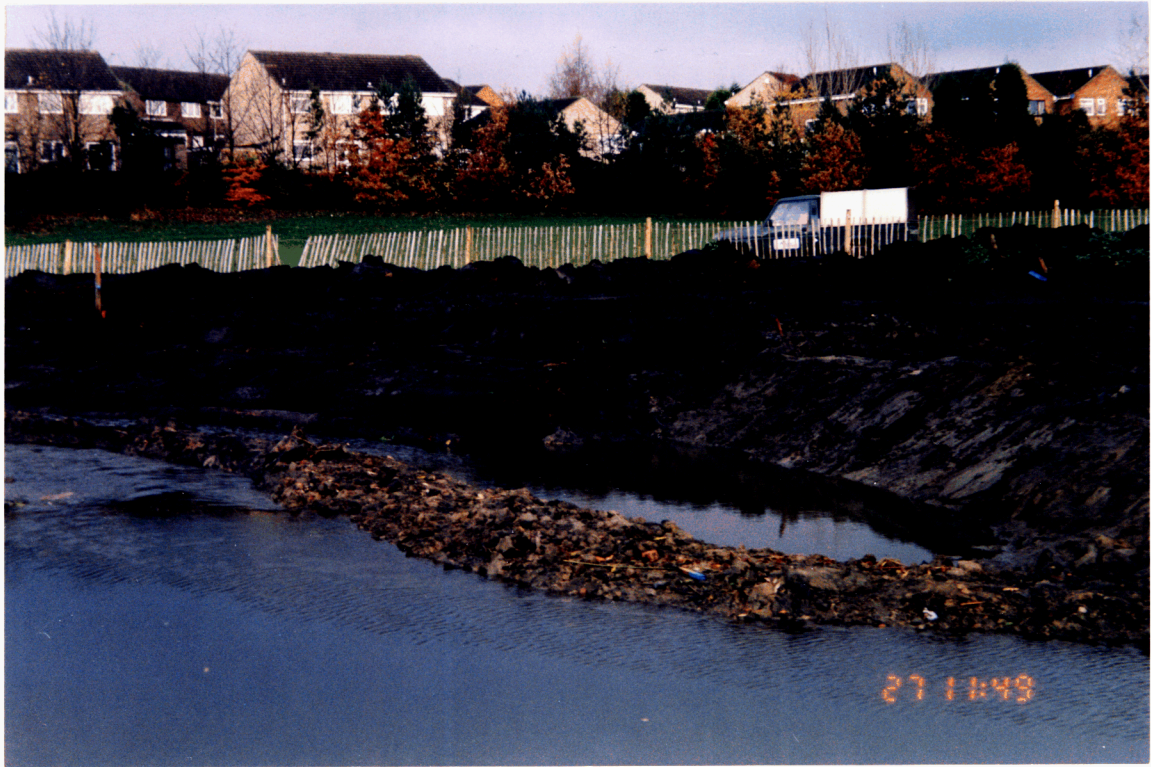
11. Log and geotextile (N3) - geotextile laid behind logs and covered with soil
