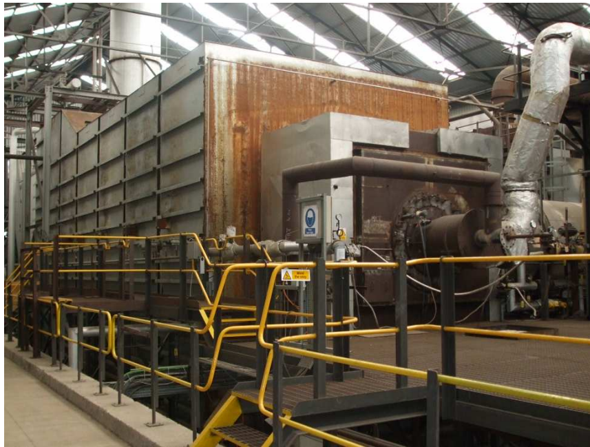
Figure 3: View of the burner gallery before upgrade for oxyfuel combustion.
