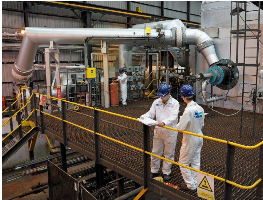
Figure 7: View of the burner gallery after upgrade for oxyfuel combustion (cf. Figure 3).
