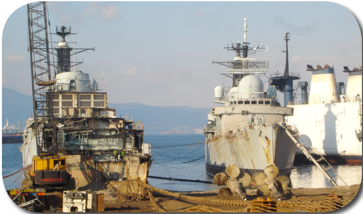
Photograph showing Nottingham & Exeter in various stages of dismantling Southampton's Propellers in the foreground
