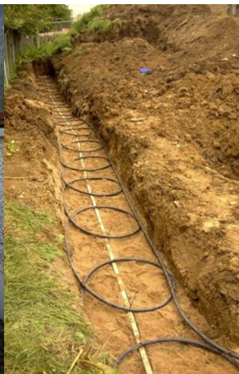
Ground Source Heat Pumps
