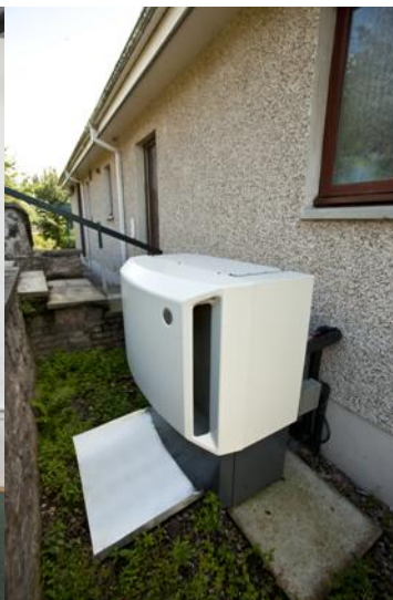
Air Source Heat Pumps
