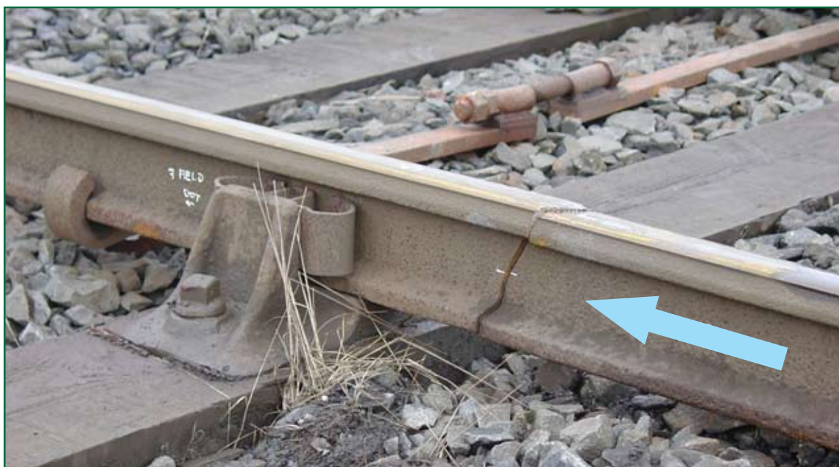
Figure 6: Rail break viewed from the field side.
