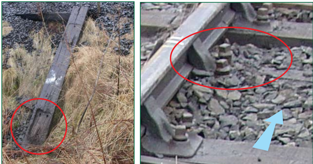
Figure 11: 45 mm indentation in sleeper preceding rail break following its removal from the track. The lack of support offered by this sleeper was significant. The displaced chairscrews and broken rail can be seen in the right hand picture.
