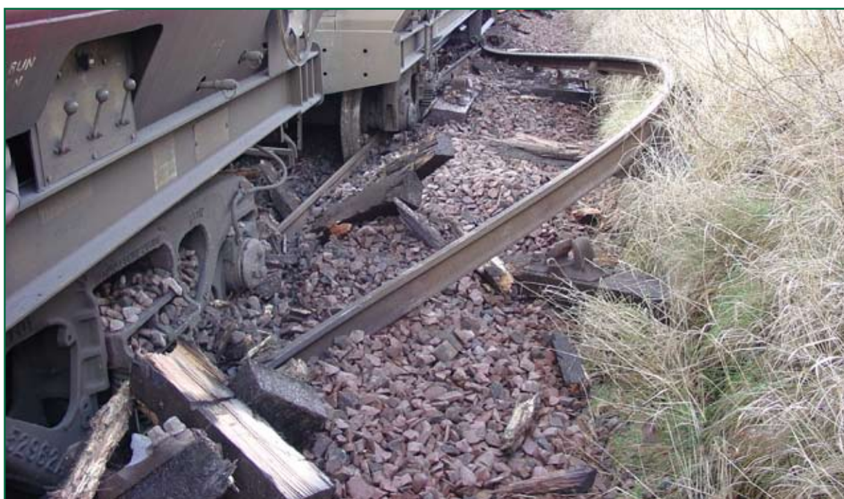
Figure 9: Derailed wagons and track damage viewed in direction of travel alongside the wagon positioned 3rd from the rear of the train. The buckled rail has been dragged forward with the train.
