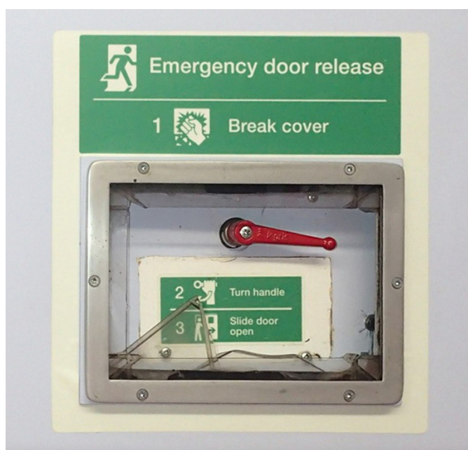
Figure 17: Emergency door release
