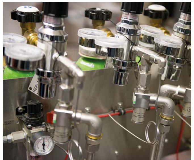
Gas control valves in the Inactive Laboratories at NNL's Central Laboratory, Sellafield
