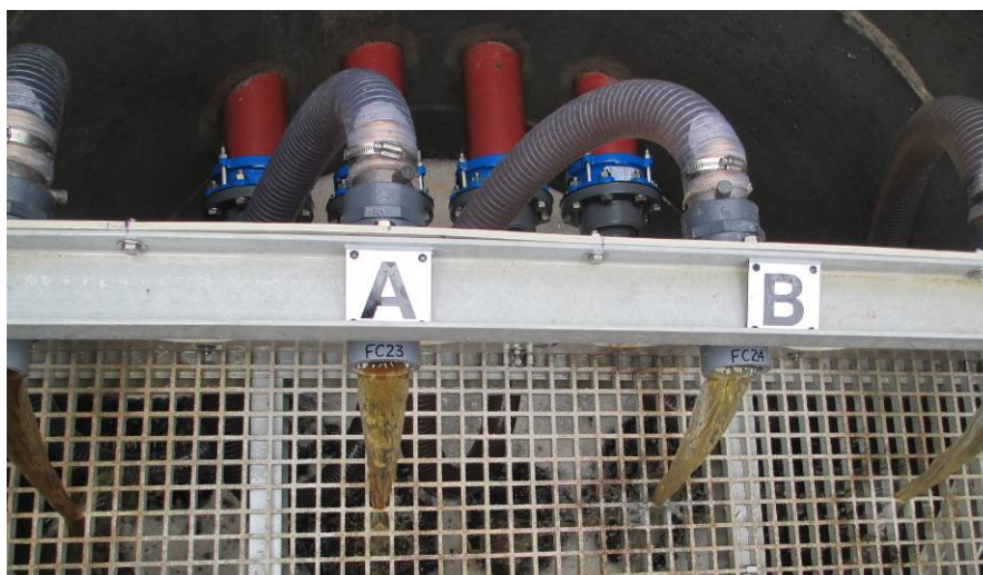
Figure 55. VFP outlet pipe arrangement at Force Crag (see text for details; note the photograph is taken less than 24 hours after system commissioning, and therefore the effluent water is temporarily discoloured) (Photograph by Newcastle University)
