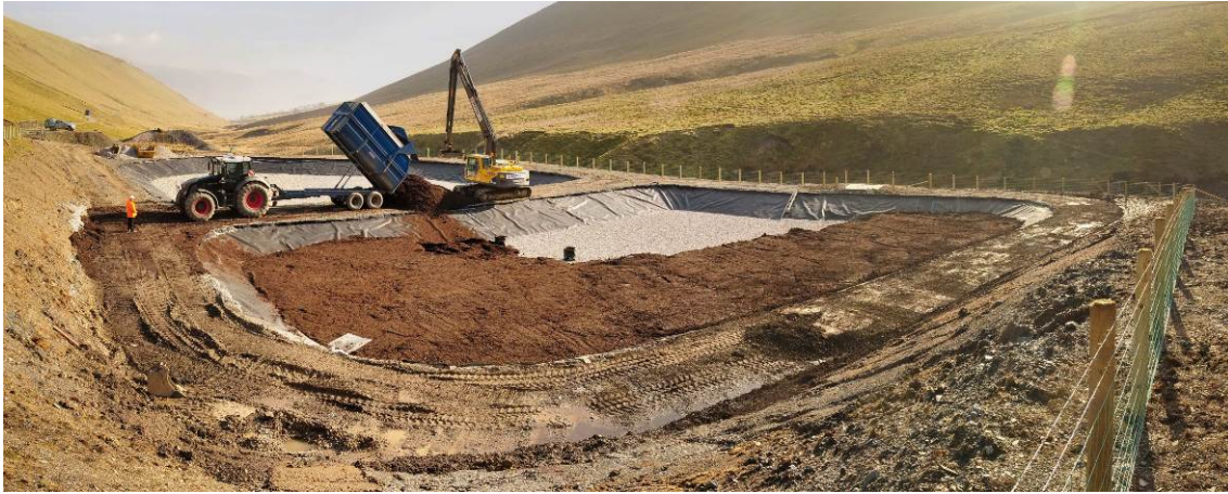
Figure 52. The two Force Crag VFPs during construction, with compost substrate being placed on top of limestone layer in VFP1 (Photograph © John Malley, National Trust)
