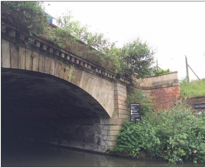
1838 section of Grade II railway bridge over Digbeth Branch Canal, into Curzon Street Station
