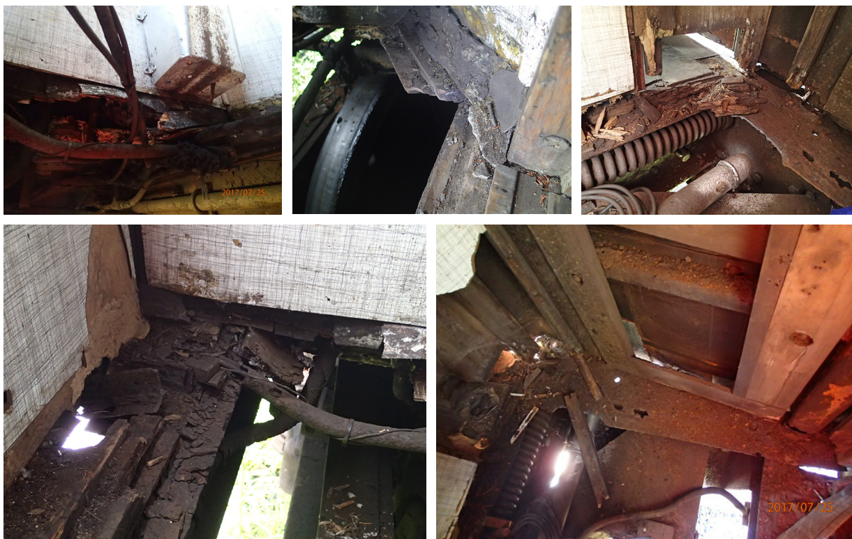
Figures 9 to 13: Details of the condition of the toilet cubicle on carriage 4805
